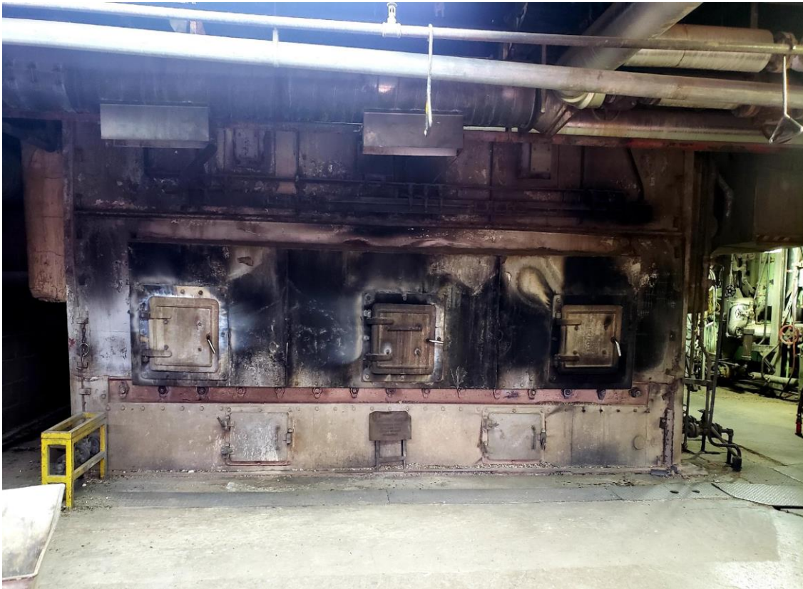
Figure 1: Incinerator Room at the Louisiana Pacific Mill in Golden.
